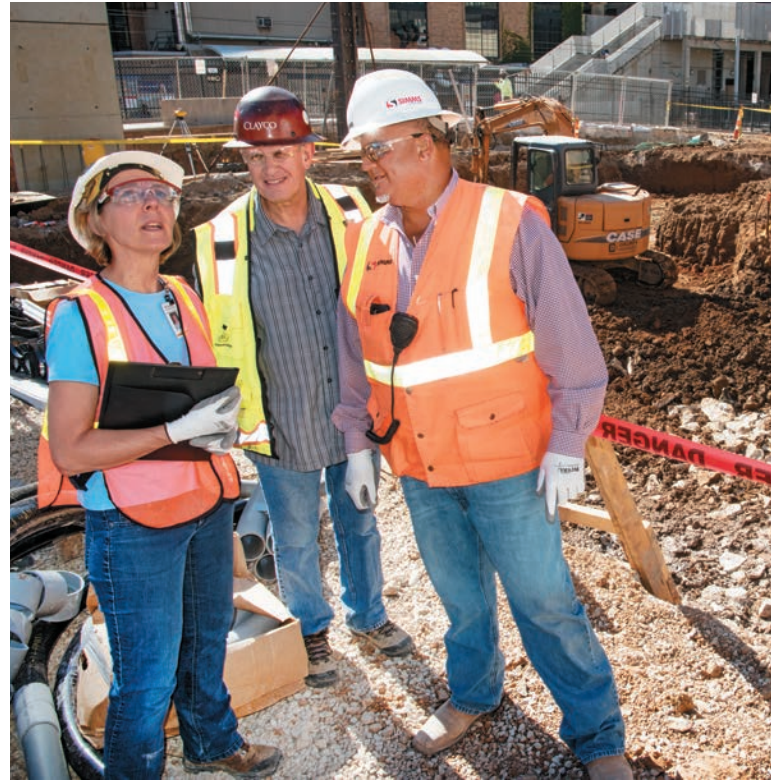
Onsite dialogue and observation have proven critical for understanding the constantly changing construction environment. Ann Marie Dale, PhD, queries Bob Hohman and Scott Sams.
